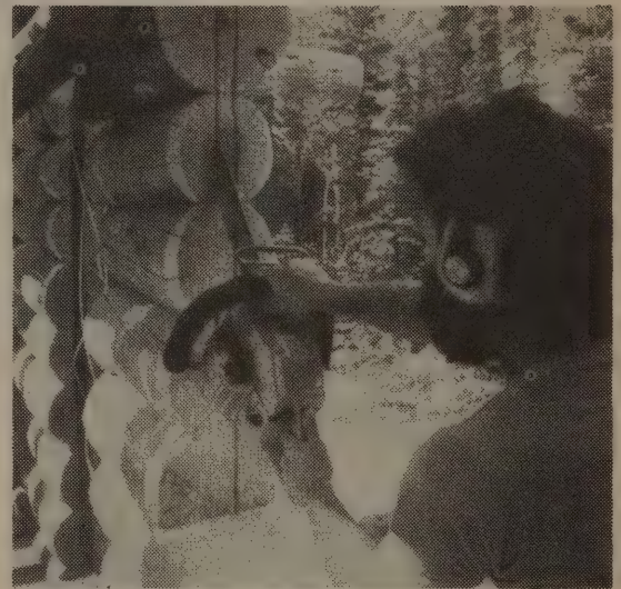
Brian Forbes splining a window. The tip of the saw is used to cut out a mortise in the window opening into which an upright 2 x 4 is placed. The cut at the upper corner is the most dangerous cut that can be made with a chainsaw on the entire project.
